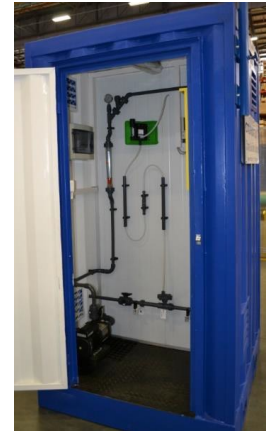
Chlorination system (Vaccuperm)
