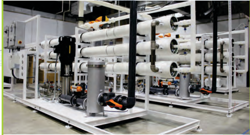
Duplex Reverse Osmosis Skids
